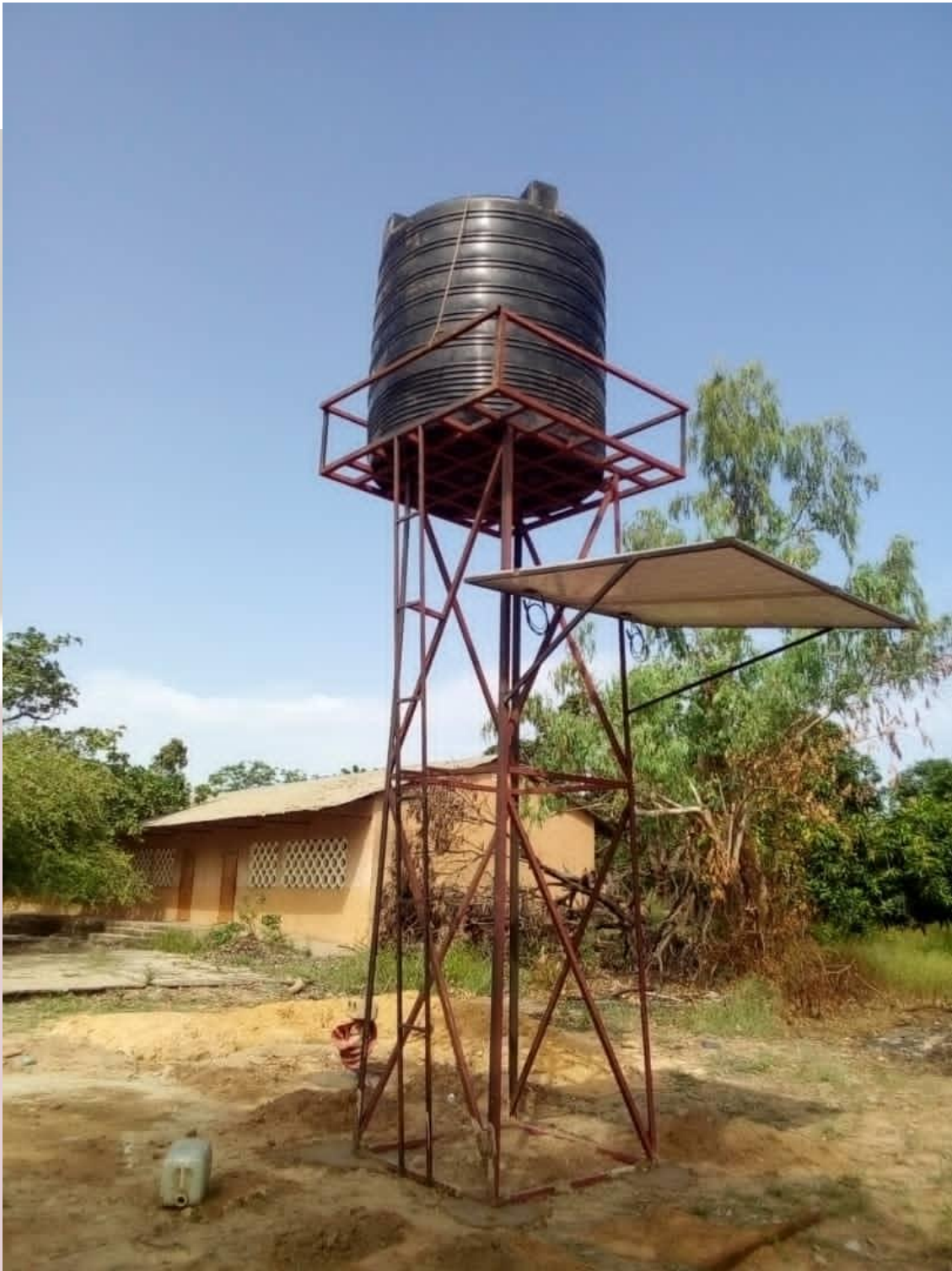
Solarwasserpumpe an der Chamen Lower Basic School
